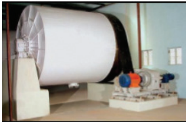
Figure 74: Conventional Ball Mill system
