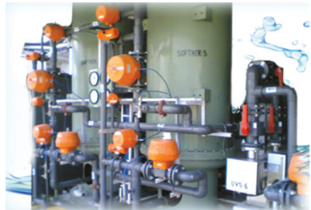
Figure 60: Water softener unit
