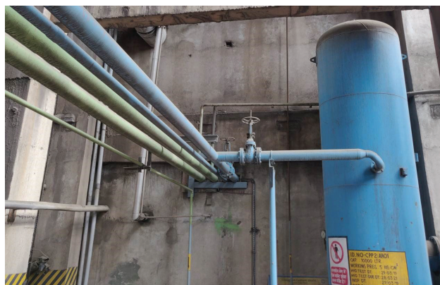
Figure 41: Existing compressed air piping
