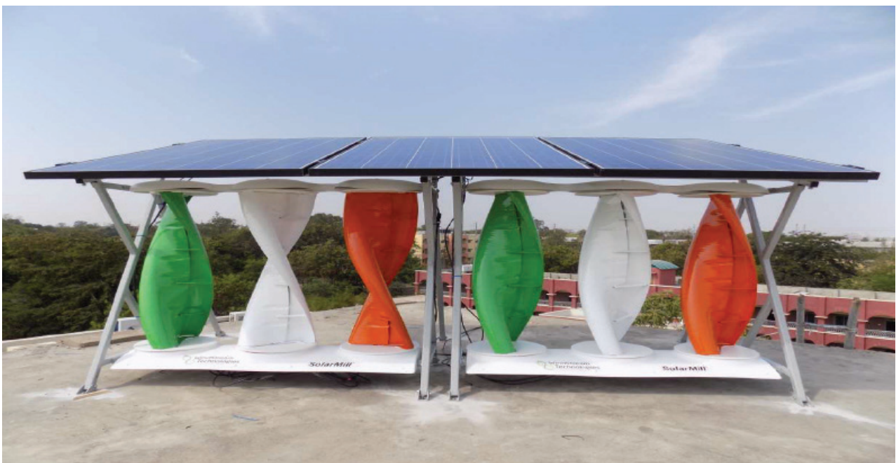
Figure 52: Solar wind hybrid system
