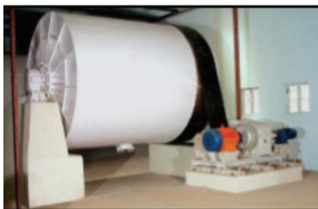
Figure 34: Conventional Ball Mill system
