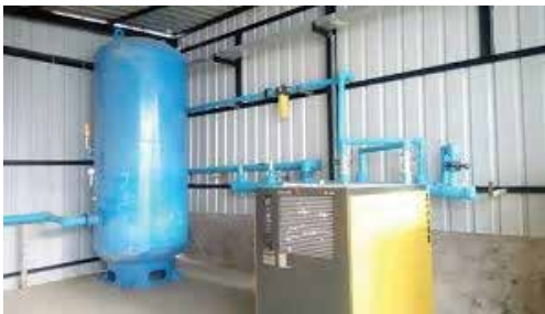
Figure 32: HDPE Aluminium Pipe line
