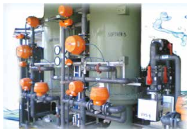
Figure 51: Water softener unit
