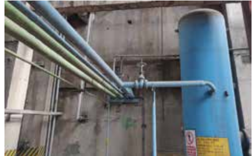
Figure 31: Existing compressed air piping
