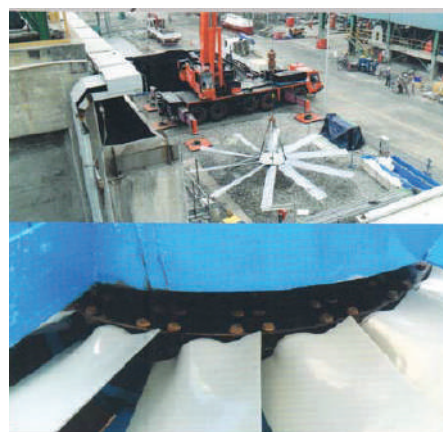
Figure 26: FRP Cooling Tower Fan
