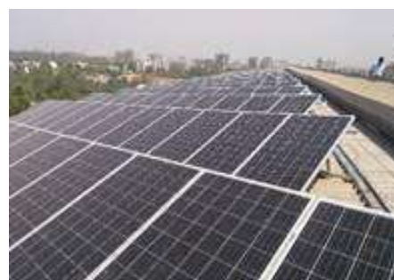
Figure 20: Solar PV Installation
